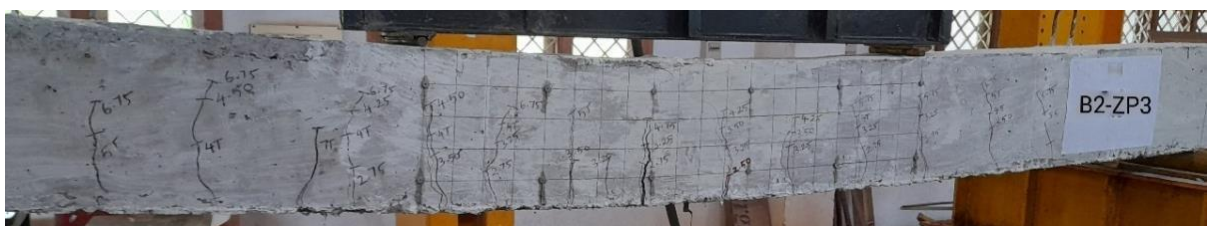
(j) Crack Pattern of B2-ZP3 Beam
