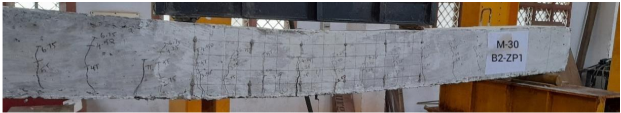
(f) Crack Pattern of B2-ZP1 Beam
