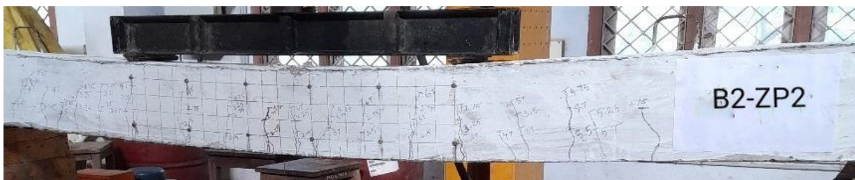
(h) Crack Pattern of B2-ZP2 Beam
