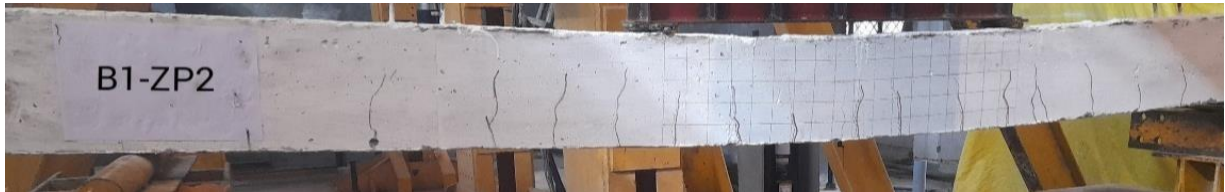
(g) Crack Pattern of B1-ZP2 Beam
