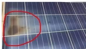
Figure 3. Typical hotspot formation in photovoltaic modules
